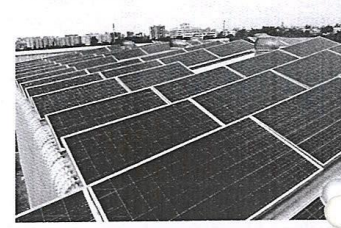
40 KWp industrial rooftop
